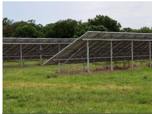
Example of a Solar Conversion System, Ground-mounted
