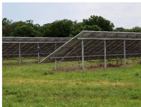
Example of a Solar Conversion System, Ground-mounted
